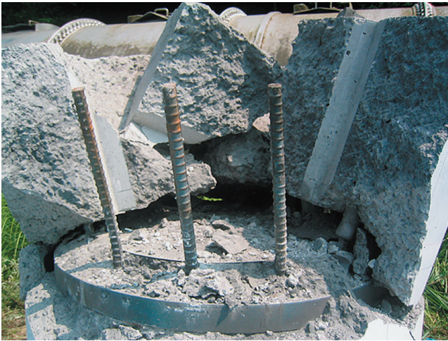
Figure 3 Fracture of the pile head by a dynamic removal method generating vertical fractures and deformation of main bars.
